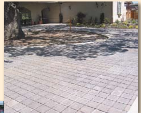
Roots feeding a 300 year-old oak tree receive additional air and water from permeable paving units at a landscape nursery in Livermore, California.
